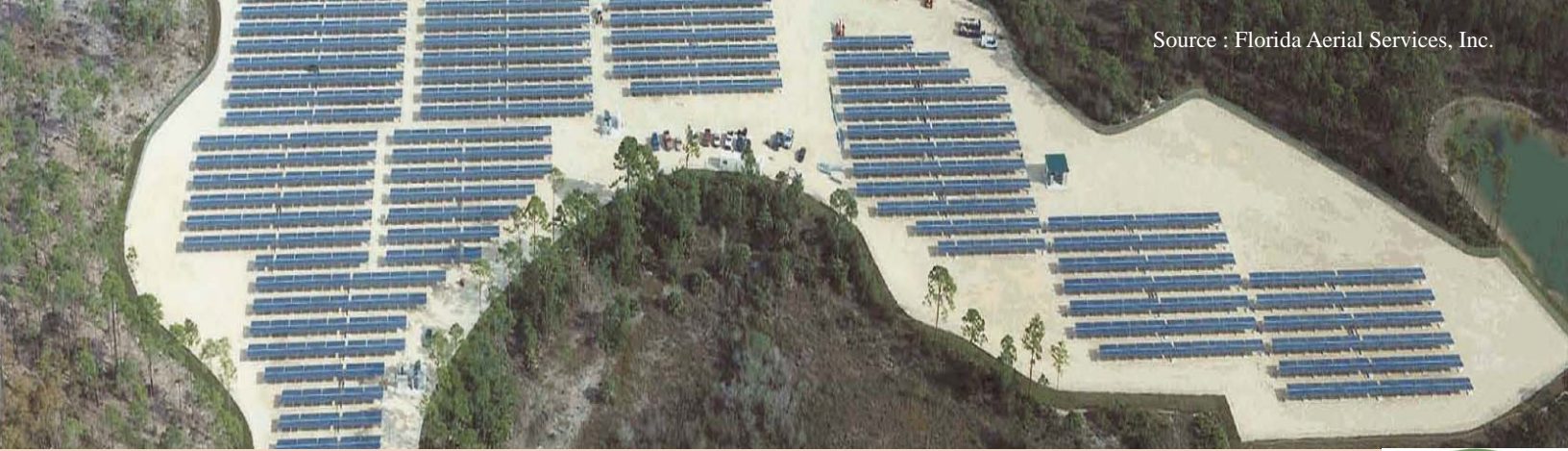
Florida Power & Light (FP&L) solar array at Florida Gulf Coast University in Lee County
